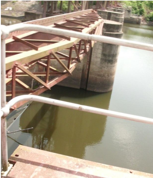
Figure 9: Weir at Iberekodo waterworks in Abeokuta
